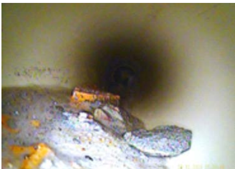
Brick and sand in sewer pipe
