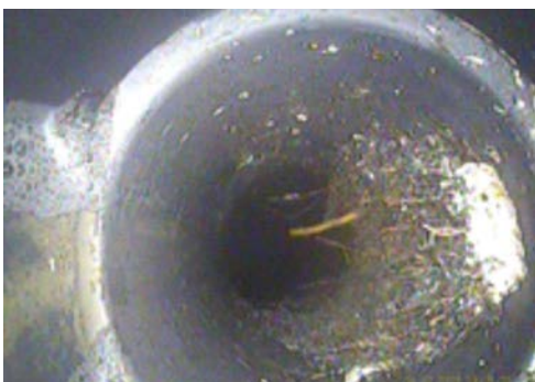
Roots in sewer pipe
